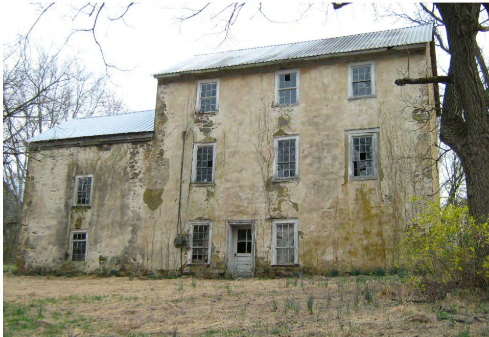
Although the 1814 stone asylum looks forlorn, much of its historic stucco remains and the building is a testament to the importance of maintaining even a basic roof, without which this building likely would be lost.
