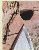
D-shaped exit hole
